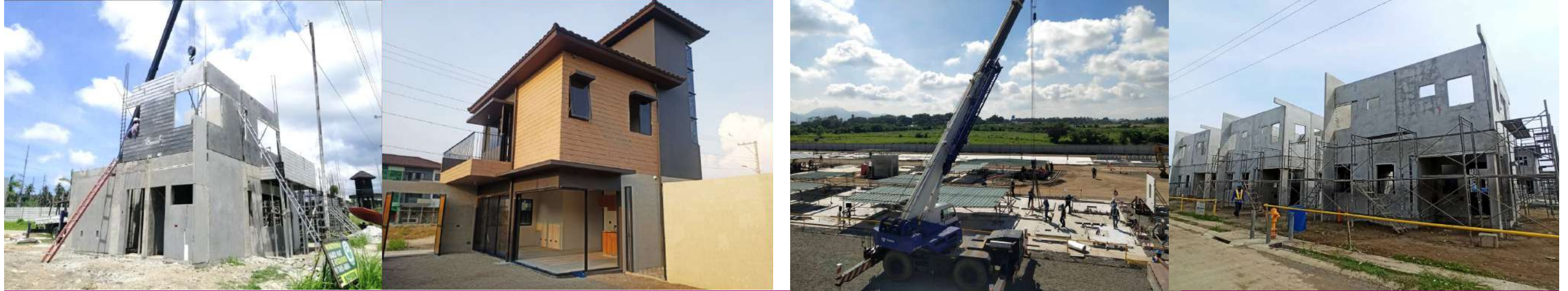
Precast technology partnerships with Sumitomo, Smart Masonry and Connovate in full swing
