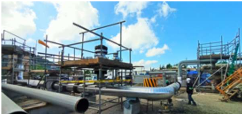
Bul 114 Wellhead Piping
