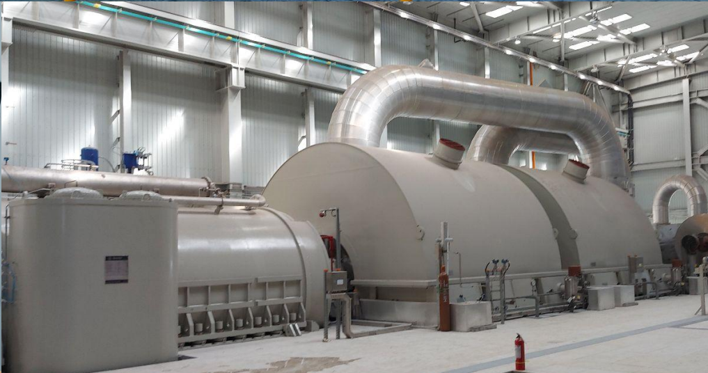
Unit 1 Steam Turbine Generator
