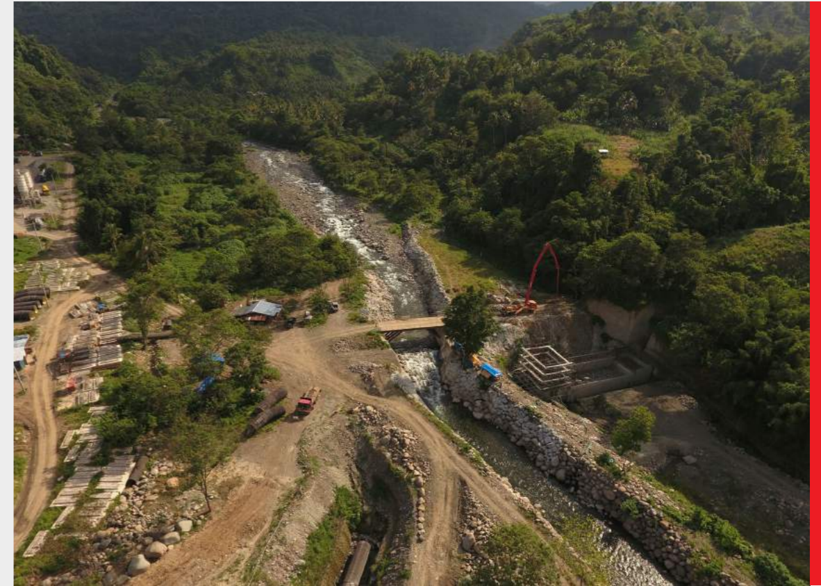
Construction continues for Apo Agua and JVACC’s bulk water supply project; above photo shows the intake weir being built at Barangay Tawantawan, Davao City
